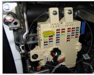
SJB (Smart Junction Box Module) Location
